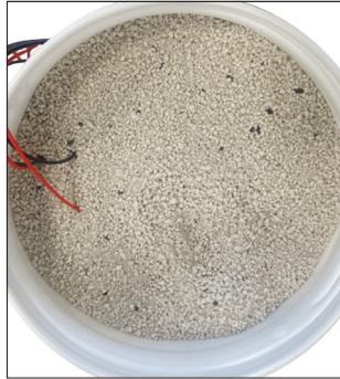
2 Loose Obexion FR poured over battery
