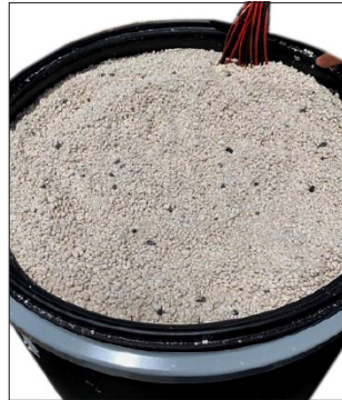
2 Loose Obexion FR poured over batteries
